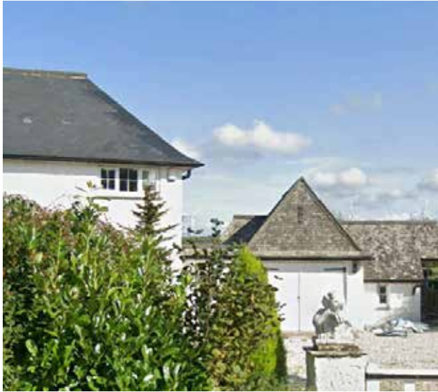
Figure 65: Notable difference in slate quality. Garage finished in quality slate with colour variation, whilst the house is matt and with uniform colour.
